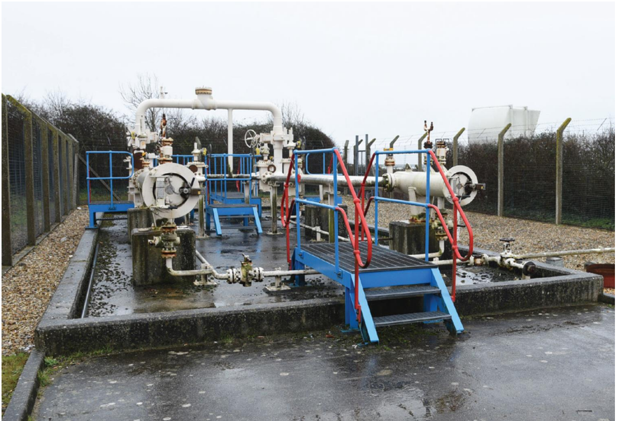
Figure 3.4 Photograph of an existing pigging station
