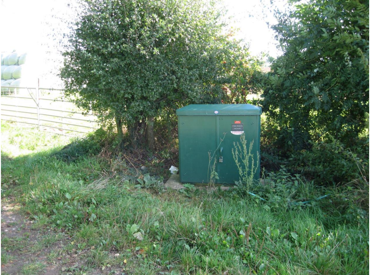
Figure 3.7 Photograph of an existing CP transformer rectifier cabinet
